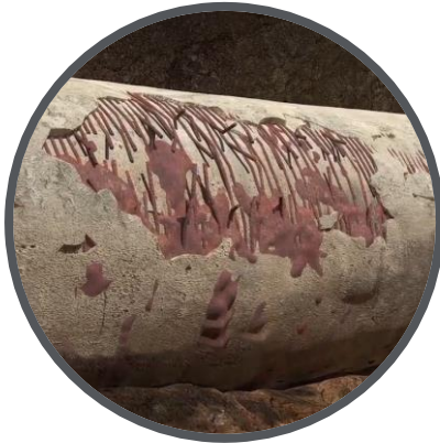
Broken bar and wire wraps
