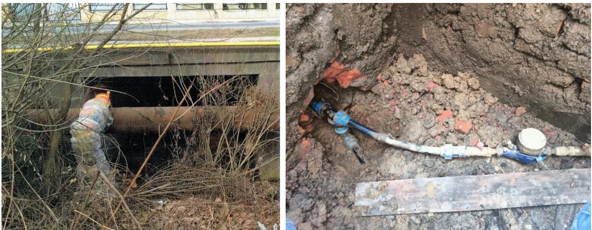
Figure. 2. Illegal connections on the water supply pipe; a – branching on the underpass pipeline of a river; b - connection on the pipe before the meter.
